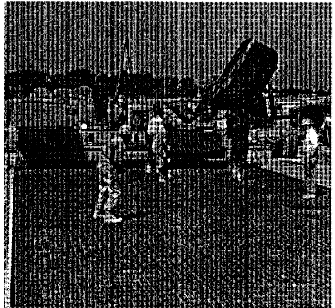
Formed concrete paving project. This is two-course work reinforcement being placed after first pass.
