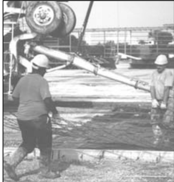
"With welded wire you don't have to prepare it — it is already welded together — you pick it up and set it in place and continue the pour" - Dave Smith, Project Manager, Murphy & Sons, General Contractor
