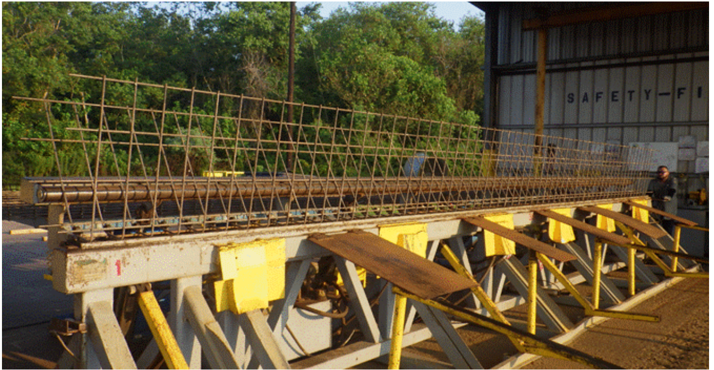
Figure 2.6: Bending Operation Step 5 – With the WWR again secured, the bending process is repeated, with the continuous rail making contact with the wires to create a pushover effect resulting in a permanent cold bend.
