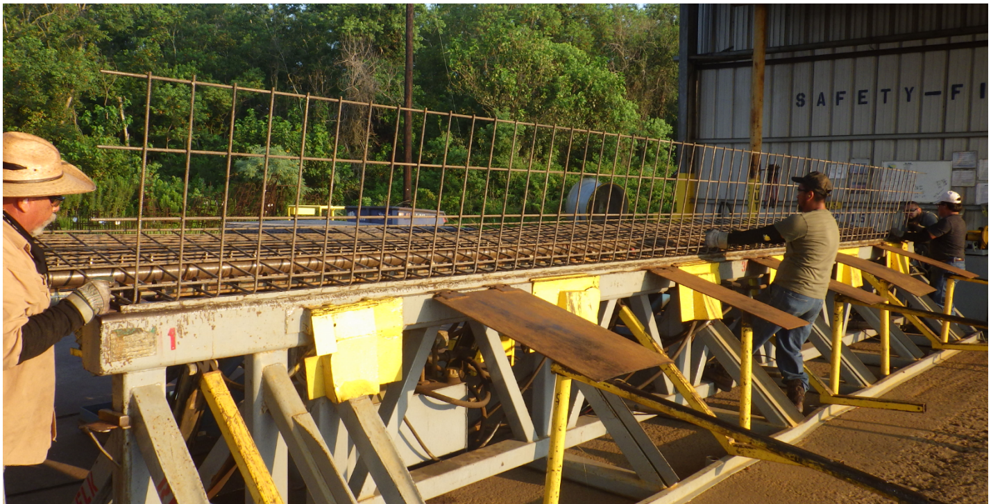
Figure 2.5: Bending Operation Step 4 – The operator resets the machine so that the continuous rail is “zero’d out”. This WWR mat is to receive two (2) 90-degree bends, so the bending crew re-position the mat so that the mandrels make contact at the precise location where the second bend is to be executed.
