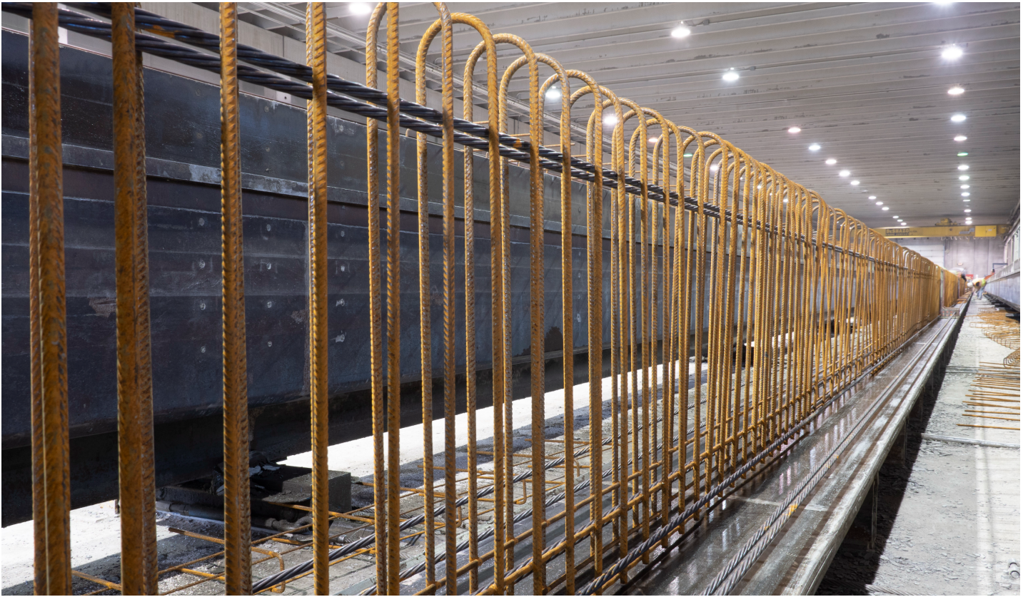
Figure 1.1: Bent WWR in a casting bed for a precast prestressed highway bridge girder
