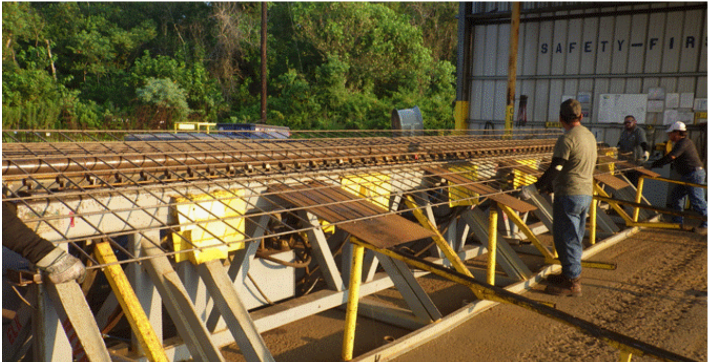
Figure 2.2: Bending Operation Step 1 – the flat WWR mat is loaded on the bender with wires to be bent aligned with the mandrels. The interchangeable mandrels are sized and spaced to suit.
