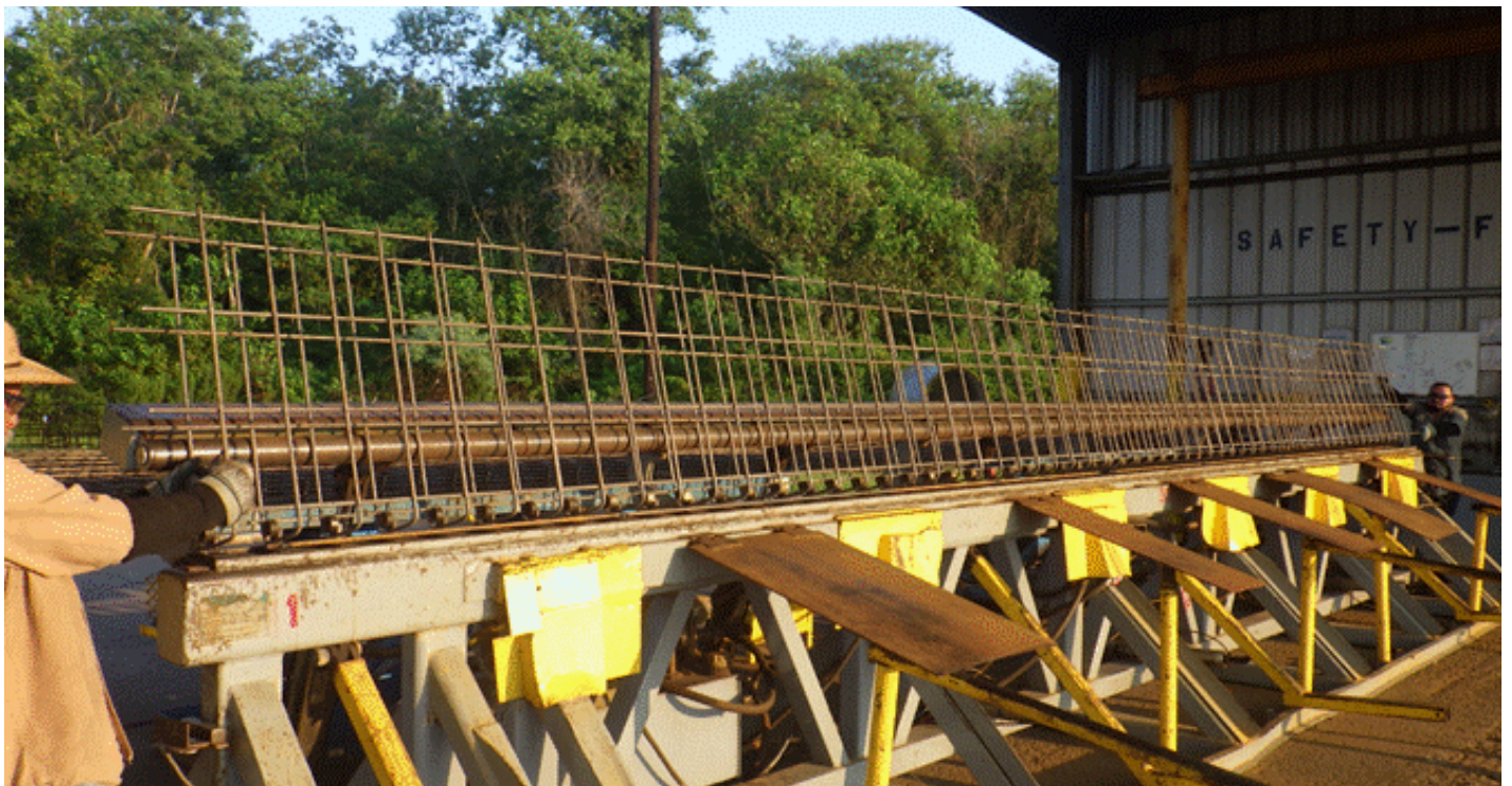
Figure 2.7: Bending Operation Step 6 – with both 90-degree angles successfully achieved, the machine is turned off and the bending crew slides the WWR mat in a longitudinal direction in order to dislodge the wires from contacting the mandrels, at which point the mat can be lifted and removed from the bender.
