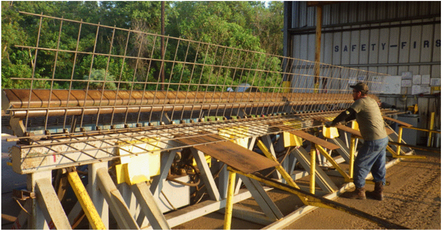
Figure 2.4: Bending Operation Step 3 – the rotation of the continuous rail terminates at the programmed angle to achieve the specified 90-degree bend angle.
