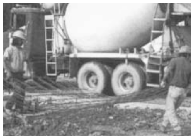
It only takes two workers to easily carry two 8'x 15' sheets of WWR, while rebar requires more expense to tie and place the material.
