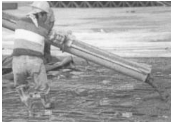
Workers walk on or into wide spaced welded wire reinforcement without deflecting or displacing it during concrete placement.
