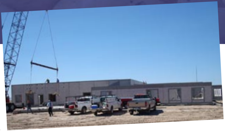
The concrete walls are being lifted into place in the laundry/bakery building. Concrete wall and roof panels are reinforced with welded wire sheets.
